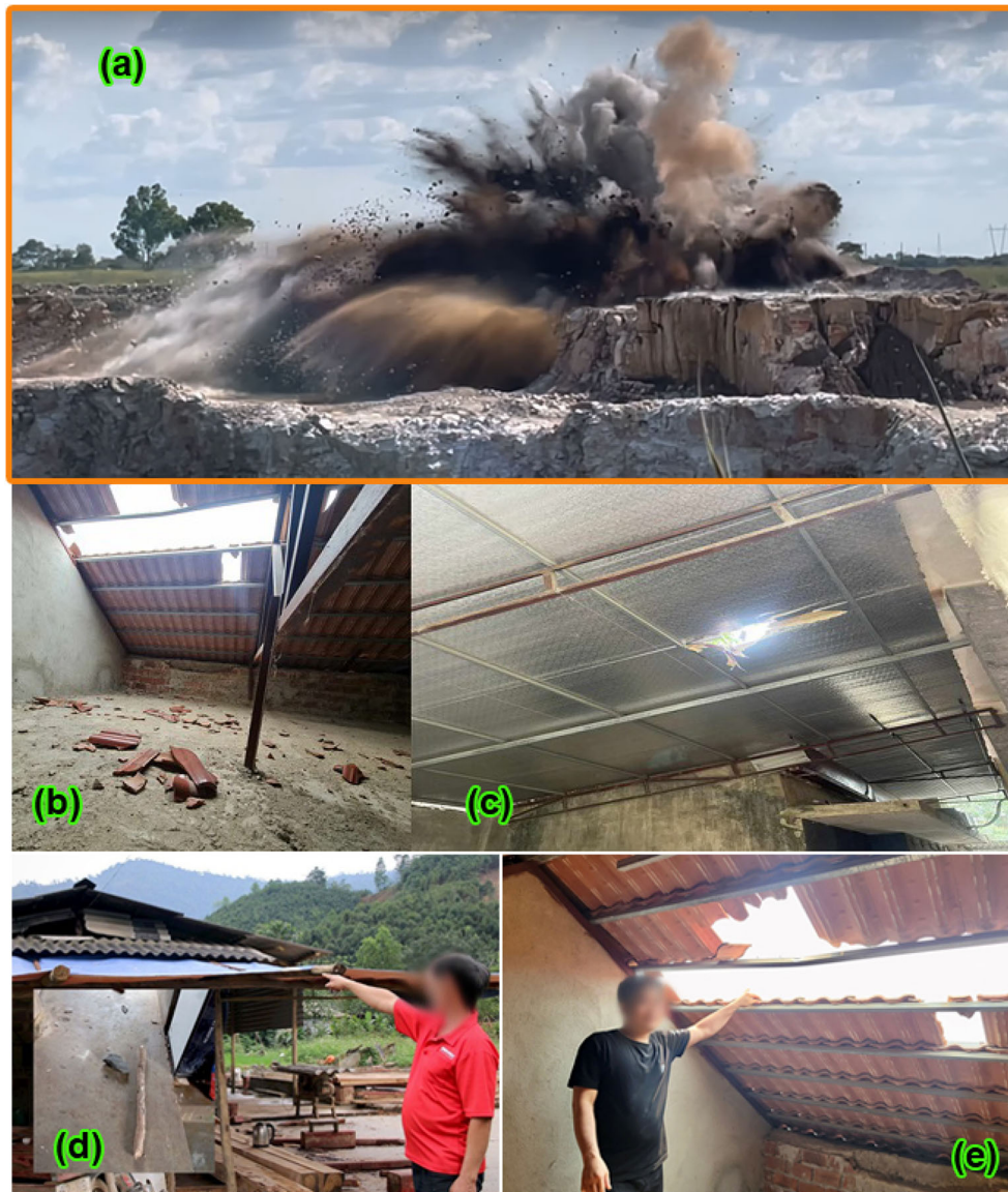
Figure 1. Blast-induced flyrock in mining and associated risks (Law, 2024; Plus, 2024): (a) flyrocks induced by mine blasting; (b)–(e) damages caused by flyrock in Vietnam.
