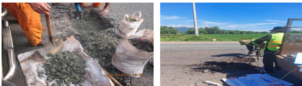
Fig. 2. Field sampling from damaged pavement a road section of National Highway 26 in Dak Lak province, Vietnam
