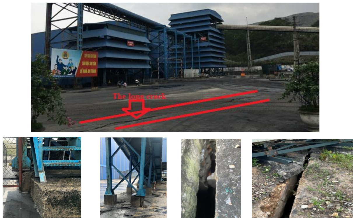
Fig. 3. The destruction of the coal storage G9, Mong Duong coal area, Quang Ninh province
