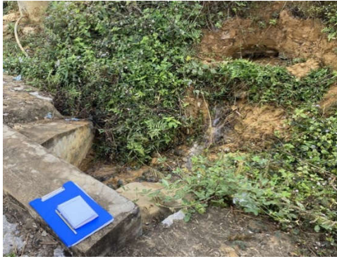
Figure 2. Seepage point with visible flow at the toe of the Dap Troi Reservoir dam (surveyed on 03/12/2021)
