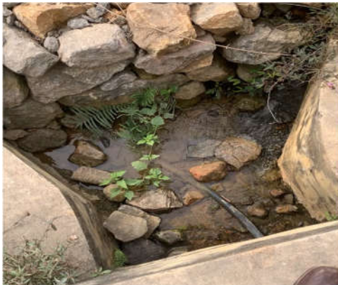
Figure 4. First seepage point at the downstream toe of Dap Troi Dam (26/12/2022); seepage persisted after slope stabilization and grouting
